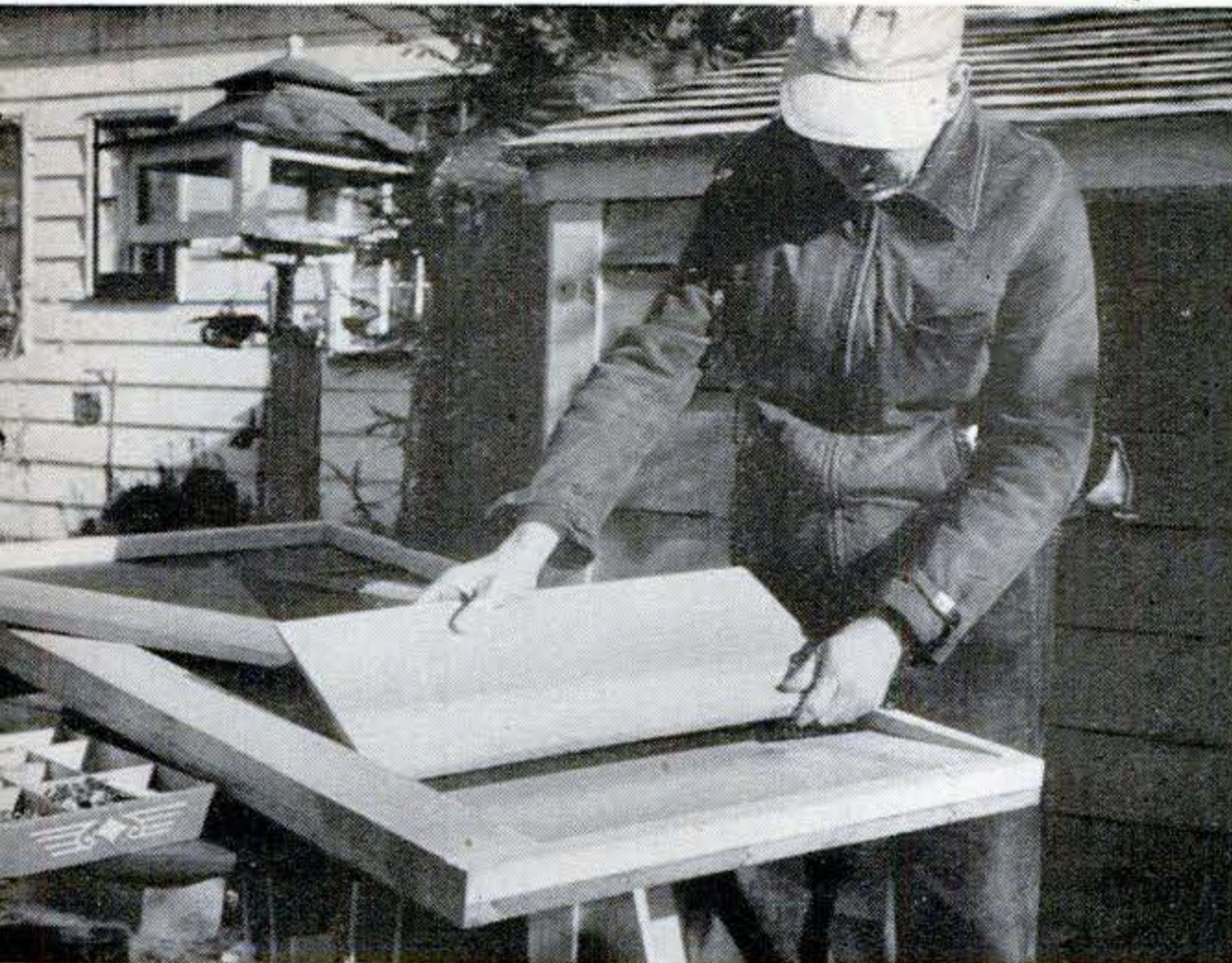
11 DOORS ARE FINISHED like walls, with tar paper, 1 1/4" edging strips and cedar siding. Add siding and last edge after you bolt or screw on the hinges.
